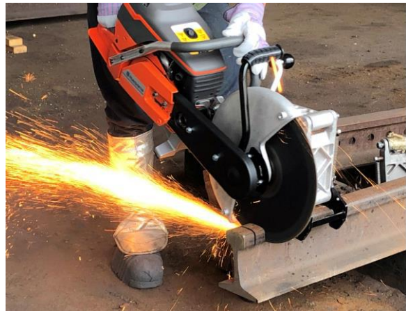
Cutting Position Inside View
